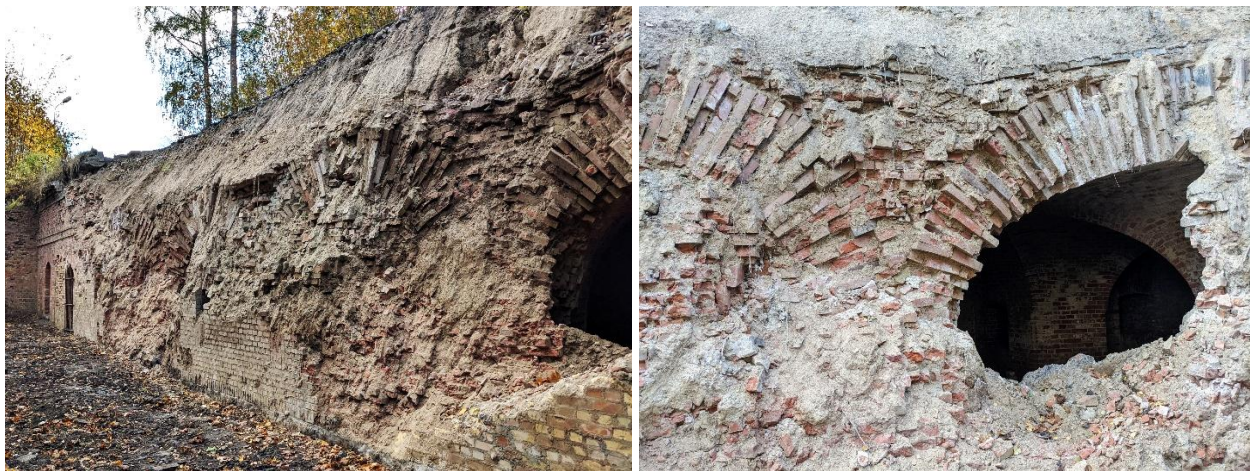
Fig. 1. Condition of the right ravelin caponier immediately after the collapse (19 July 2022).
